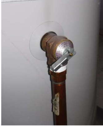
Water heater temperature pressure relief valve
