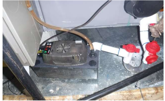
A condensation pump for an air conditioning system in a catch pan.
