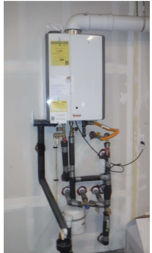
Typical tankless water heater installation
