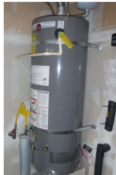
A properly strapped water heater
