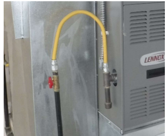
A properly configured gas line, shut off valve, and drip leg
