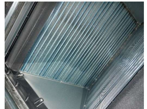
An evaporator, located inside the air handler system
