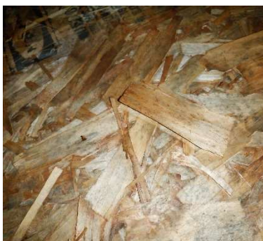
Moisture-stained roof sheathing, dark spots can be seen on the wood
