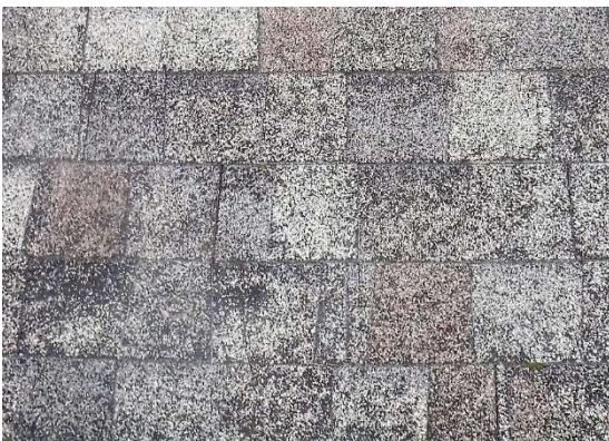
Roofing with missing granules
