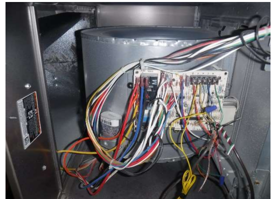
A furnace air handler
