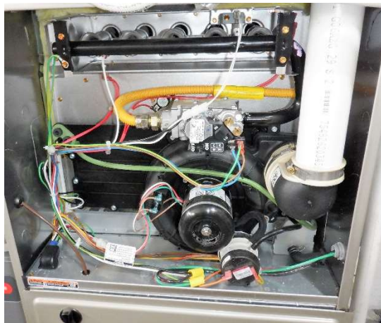
A high efficiency furnace, note the back plastic area around the induction fan and the plastic exhaust flue pipes
