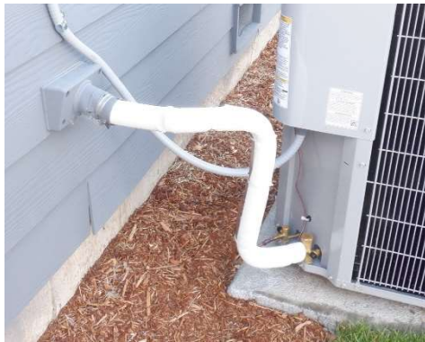
Insulation around the low pressure gas line of the A/C system
