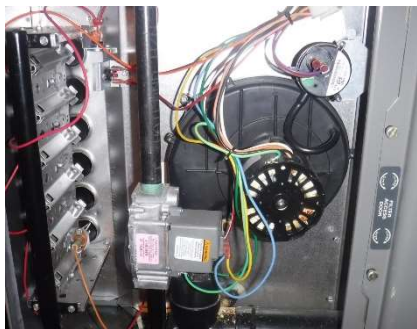
The draft induction fan motor, the motor is centered in the back circle.
