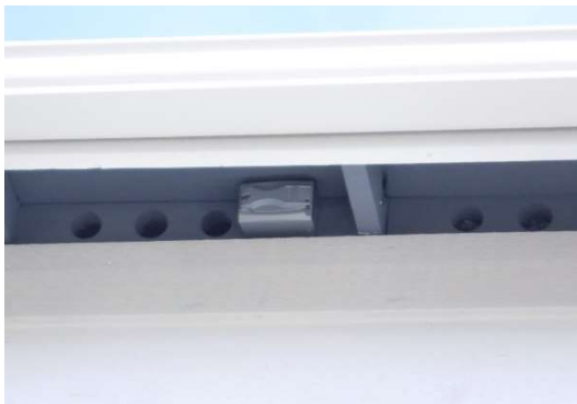
Bird block style lower roof vents, an electrical outlet for Christmas lights can be seen.
