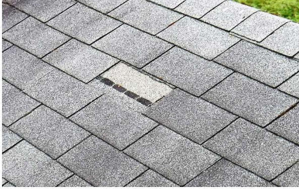
Missing tab from Three-tab shingles, Note the black adhesive strip on the lower shingle
