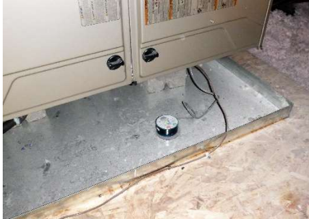
A condensation catch pan and sensor under a high efficiency furnace
