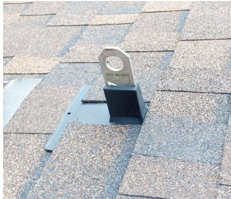
Roof anchor missing its protective cap
