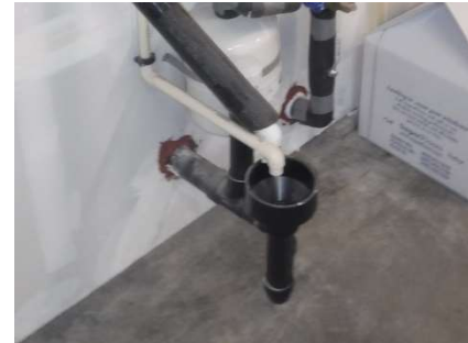
A CPVC TPRV discharge pipe draining into an ABS waste pipe
