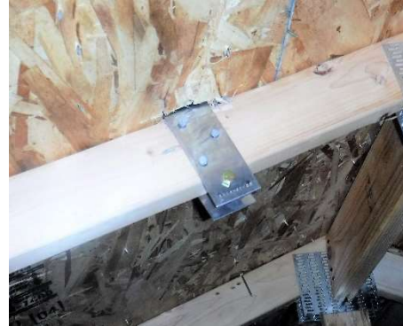
This tie off penetration is a common areas roof leaks are seen
