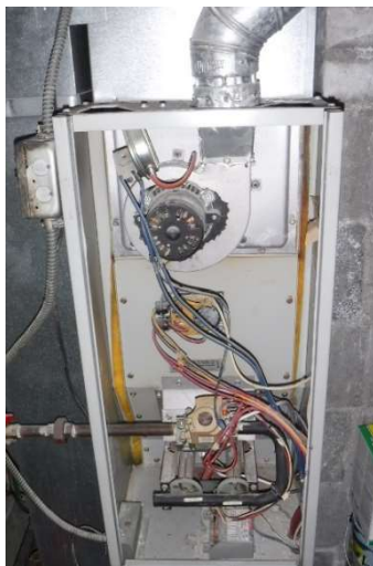
An older mid efficiency furnace
