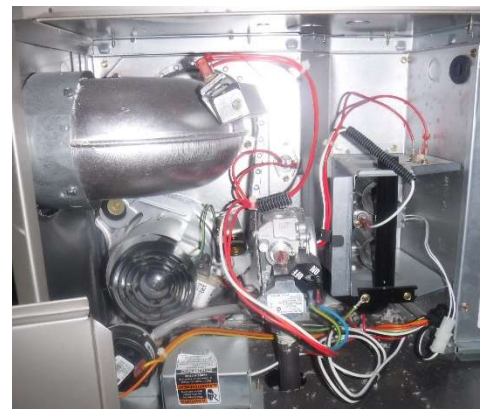
A mid efficiency furnace, note the metal flue pipe
