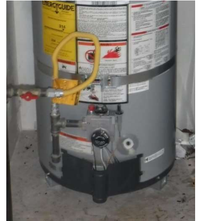
A flexible gas line with drip leg and shut off valve
