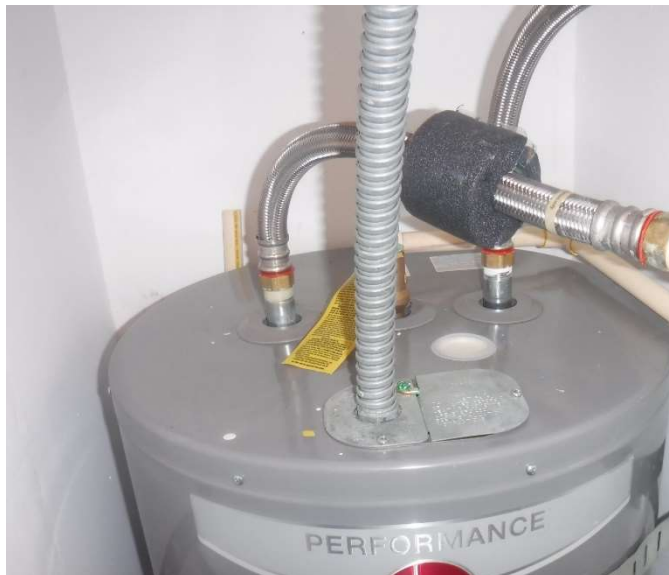
Armored cable run to an electric water heater
