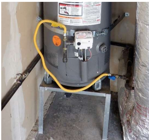
An elevated FVIR water heater
